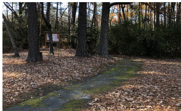
Nike Park – Sidewalks are cracked and overgrown, limited ADA accessibility
