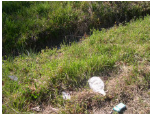
This ditch will carry roadside litter, as well as nutrient pollution from fertilizers, into streams and rivers and ultimately into the Chesapeake Bay.
