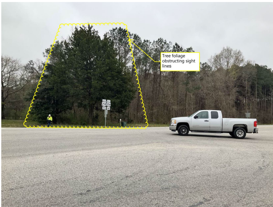
Figure 9. Tree foliage obstructing sight lines between through vehicles on Scotts Factory Road and turning vehicles on Courthouse Highway
