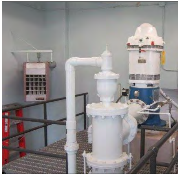
Inside of Well #4
