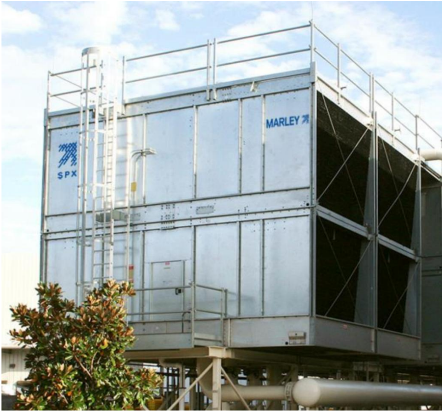
Cooling Tower (dual cell)
