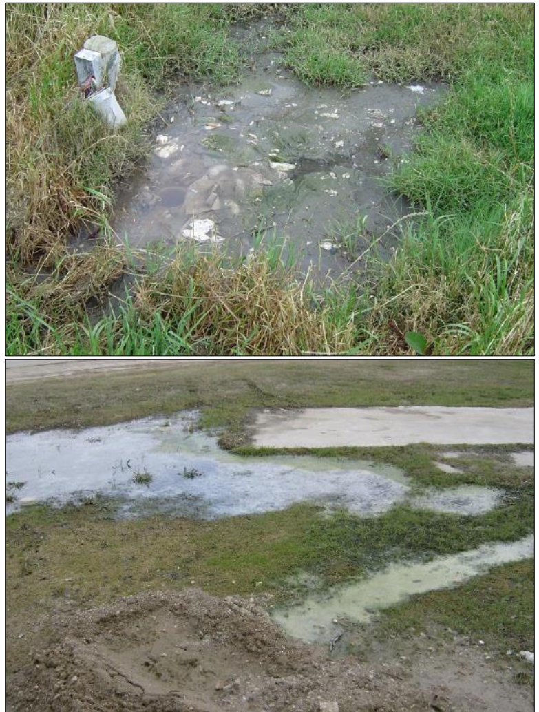
OSSF malfunctions can occur due to lack of maintenance, improper construction in unsuitable soils, or overloading the drain field, resulting in overflows at the surface (City of Arlington).
