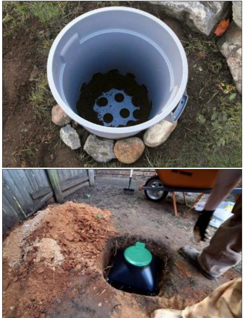
Above: Installation of DIY pet waste digester (Zach Ogilvie, www.instructables.com ). Below: Installation of prefabricated pet waste digester near Lake Arlington.
