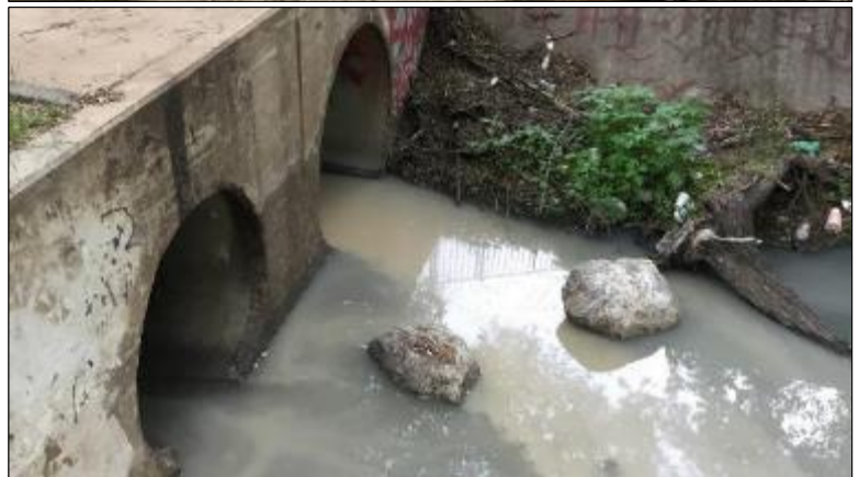
Above: Active SSO with flow from sewer access (credit: City of Arlington). Middle: Evidence of recent wet-weather SSO – note debris around rim (credit: City of Fort Worth). Below: Underground SSO, emerging at a culvert (credit: City of Fort Worth).
