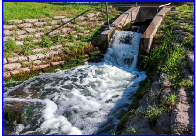
Fig. 3c. Outfall of TRA's Red Oak Creek Regional Wastewater System
