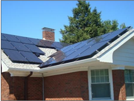
Roof Mounted Solar
