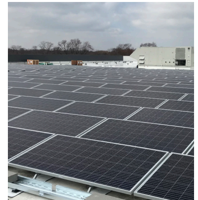
Municipal Solar Panels
