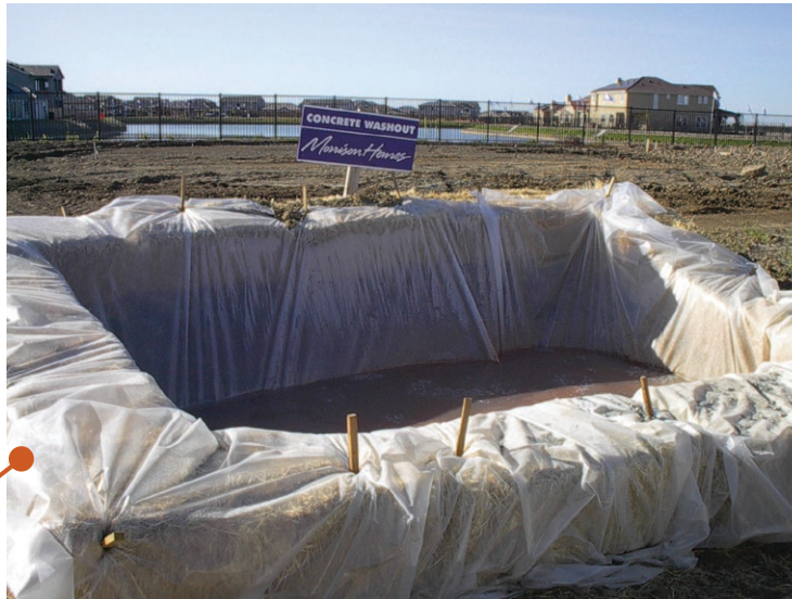
Photo 1: Well-maintained and labeled concrete truck washout
