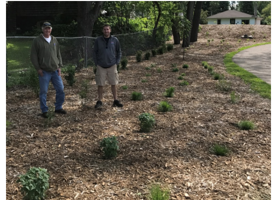
Public Works Workers Kurt Siebert and Nick Kleve finish some natural landscaping and pollinator garden installation in Monroe Park.
