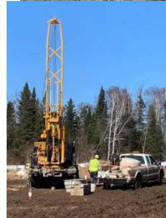
Left: Enbridge contractors on the shores of the Mississippi River preparing to take core samples for Horizontal Drilling underneath the river
