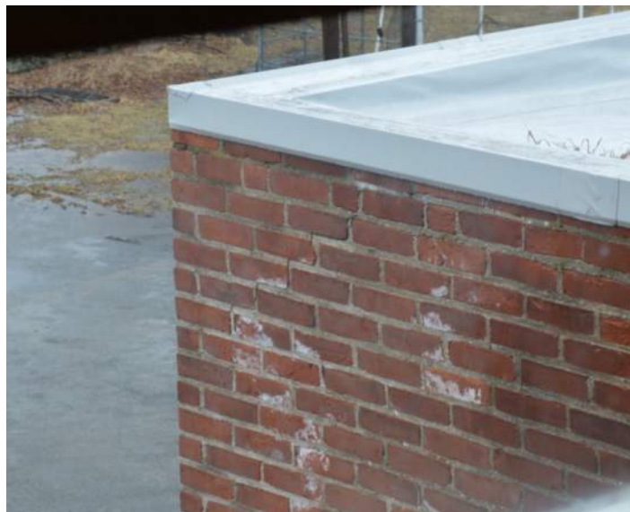
Photo 23: Stress Crack in the Masonry Wall, Rear Facade.
