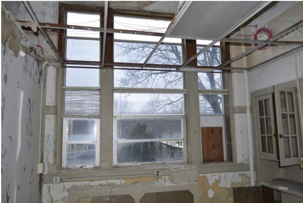
Photo 13: The height of the window openings has been obscured by a lowered ceiling, changing the proportions of the classroom and office spaces, and limiting natural lighting. The original ceiling height should be maintained. Original cabinetry should be retained to the greatest extent possible.
