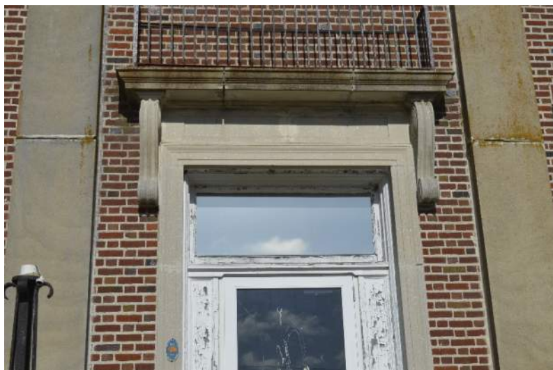
Photo 25: Horizontal joints at the pilasters need repointing as do the vertical joints in the hood over the front door.
