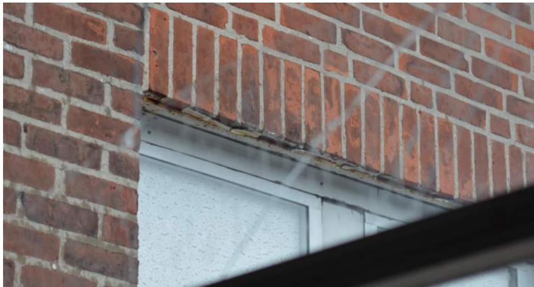
Photo 21: Corroded Steel Lintel over Window
