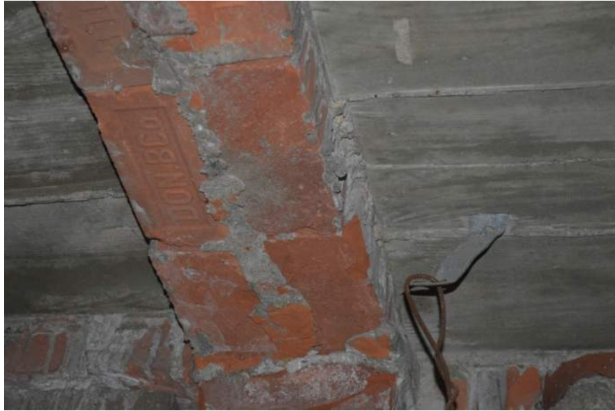
Photo 20: Unsupported Brick over Newer Elevator Opening
