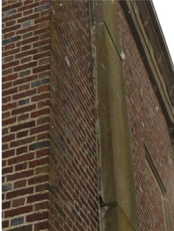
Photo 22: Cast Stone Ornamentation Shifting, Front Facade
