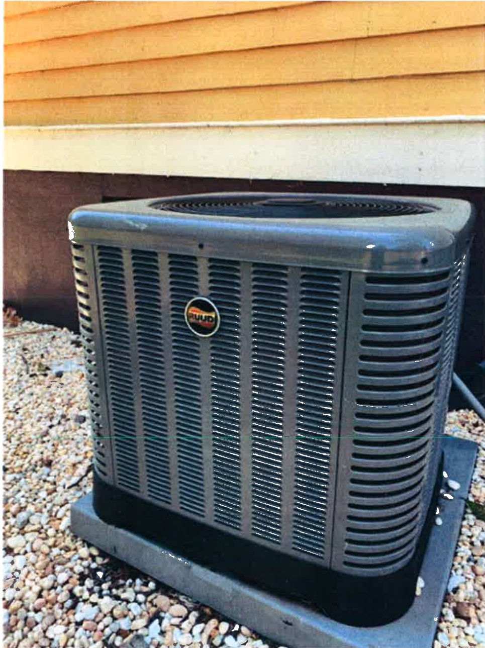
HVAC UNIT 1 No Longer Visible Due TO 6' PROPOSED Fence
