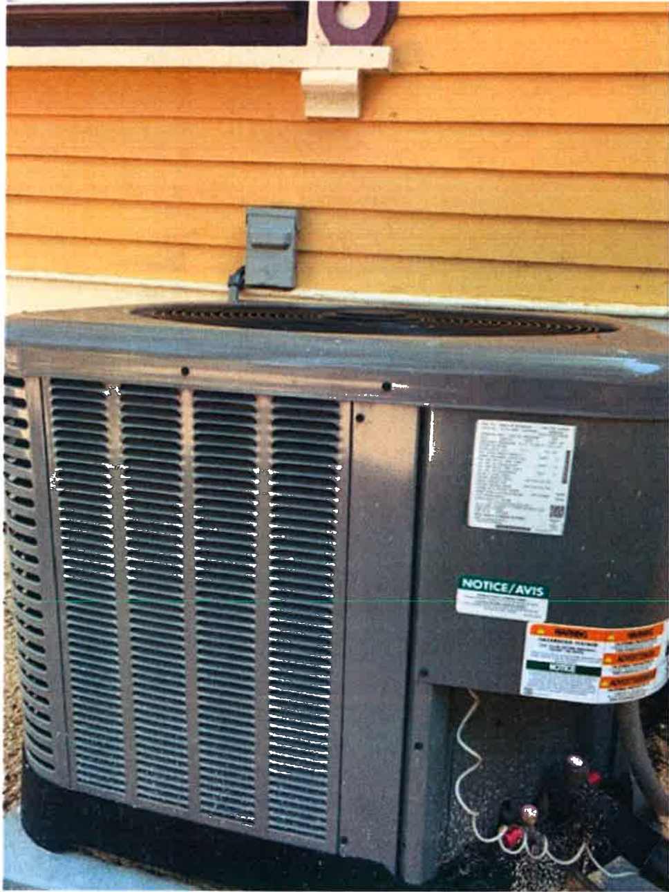
HVAC UNIT 2 - Not Visible
