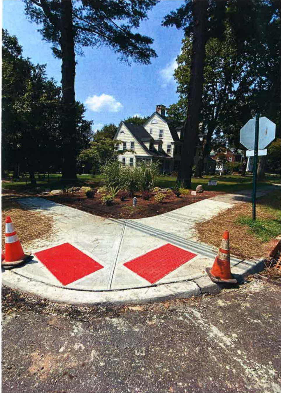
CORNER OF HILLSIDE AND PROSPECT AVENUE AFTER SIDEWALK CONSTRUCTION. PROPOSED LOCATION OF BLUESTONE WALL.
