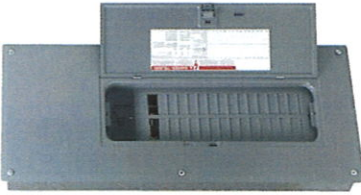
Main Service Panel
