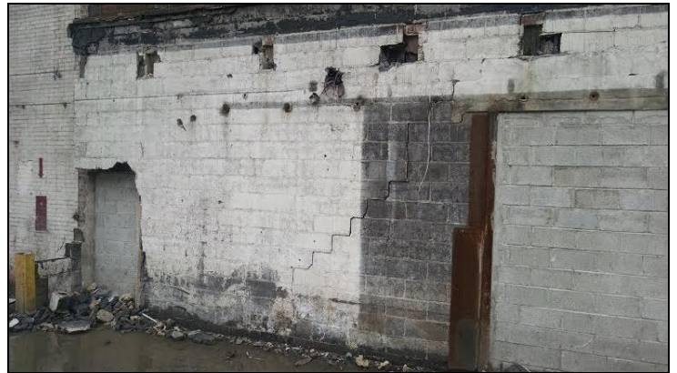
Evidence of structural damage to cinder block wall
