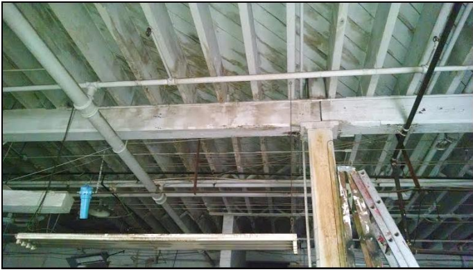
Water damage to ceiling
