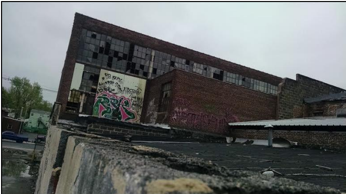
Broken windows, dilapidated building, graffiti
