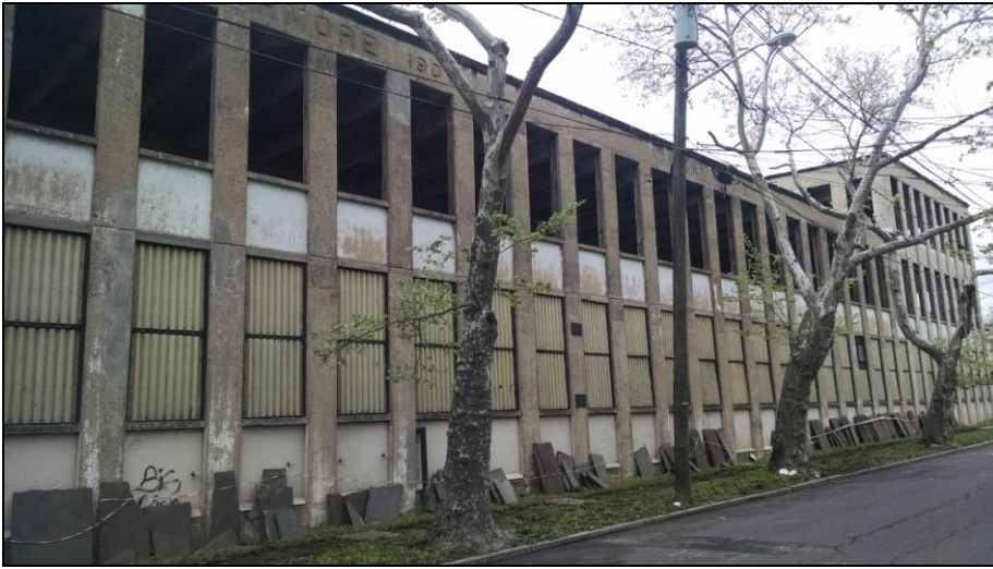
Front elevation of 639-661 South Avenue “Royal Apex Building” along South Avenue (flagstone sidewalks being salvaged)
