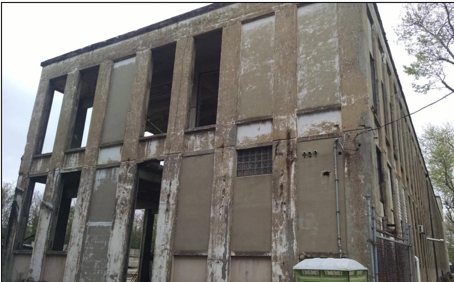
West elevation of 639-661 South Avenue “Royal Apex Building” demolition work in progress
