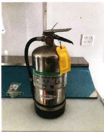
"K" Class Extinguisher
