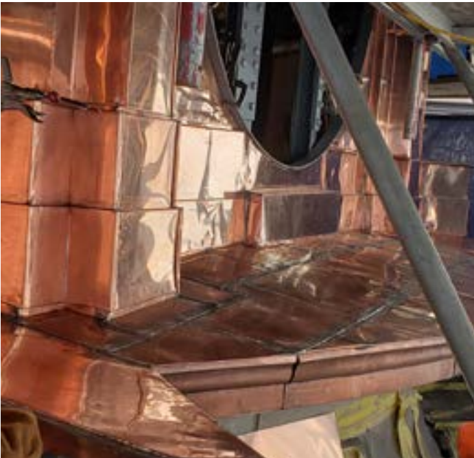
Copper work at the clock dial base. There are four similar areas like this to repeat the work on. Due to the original construction, each one is slightly different in size.
