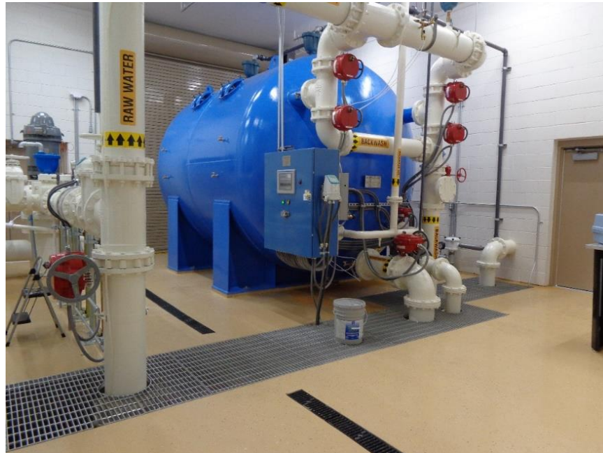
Figure 18: Manganese pressure filtration system.
