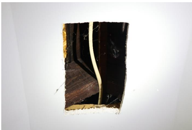
Figure 9. WJE conducted inspection opening 5 in the Second Level ceiling to observe the roof ridge beam.
