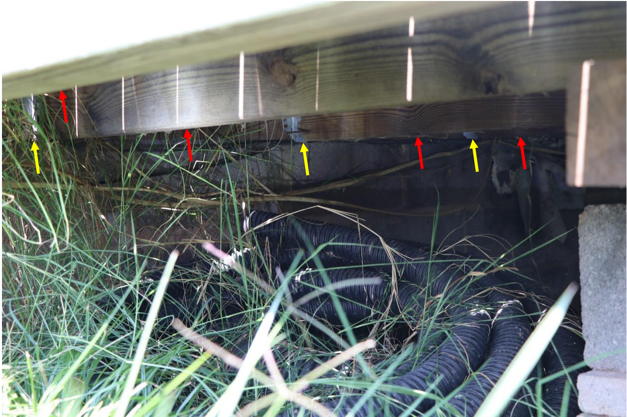
Figure 14. The front porch consisted of pressure treated wood (red arrows) supported metal joist hanger (yellow arrows) at the Cottage facade.
