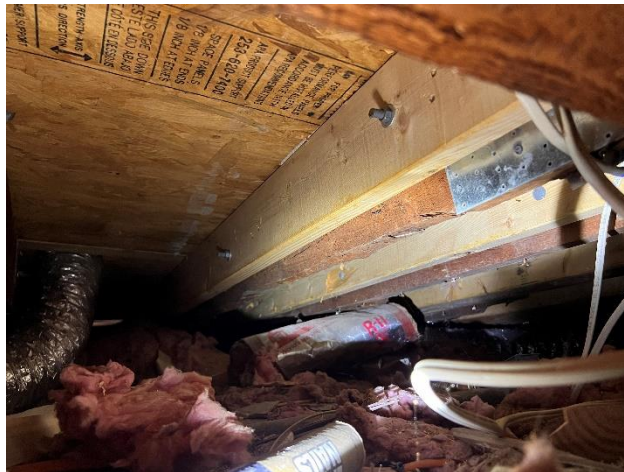
Figure 8. WJE conducted inspection opening 4 in the stairwell wall to observe the Second Level framing.
