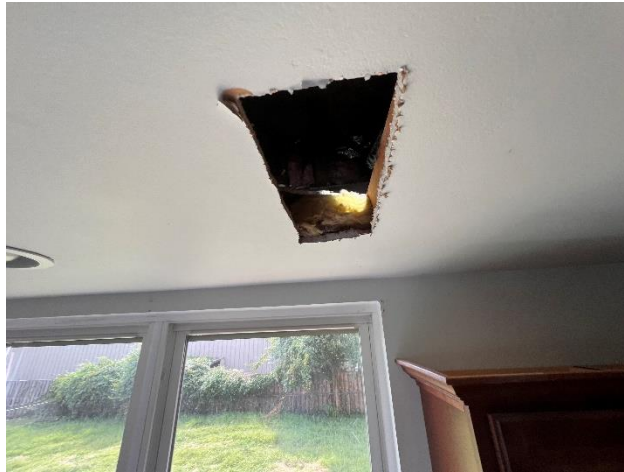
Figure 6. WJE conducted inspection opening 2 in the kitchen ceiling to observe the Second Level framing.
