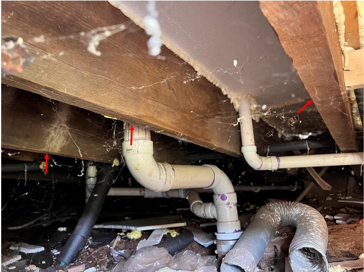
Figure 24. The First Level floor joists (red arrows) measured 2-inches wide by 10-inches deep and were spaced at 16-inches on-center.
