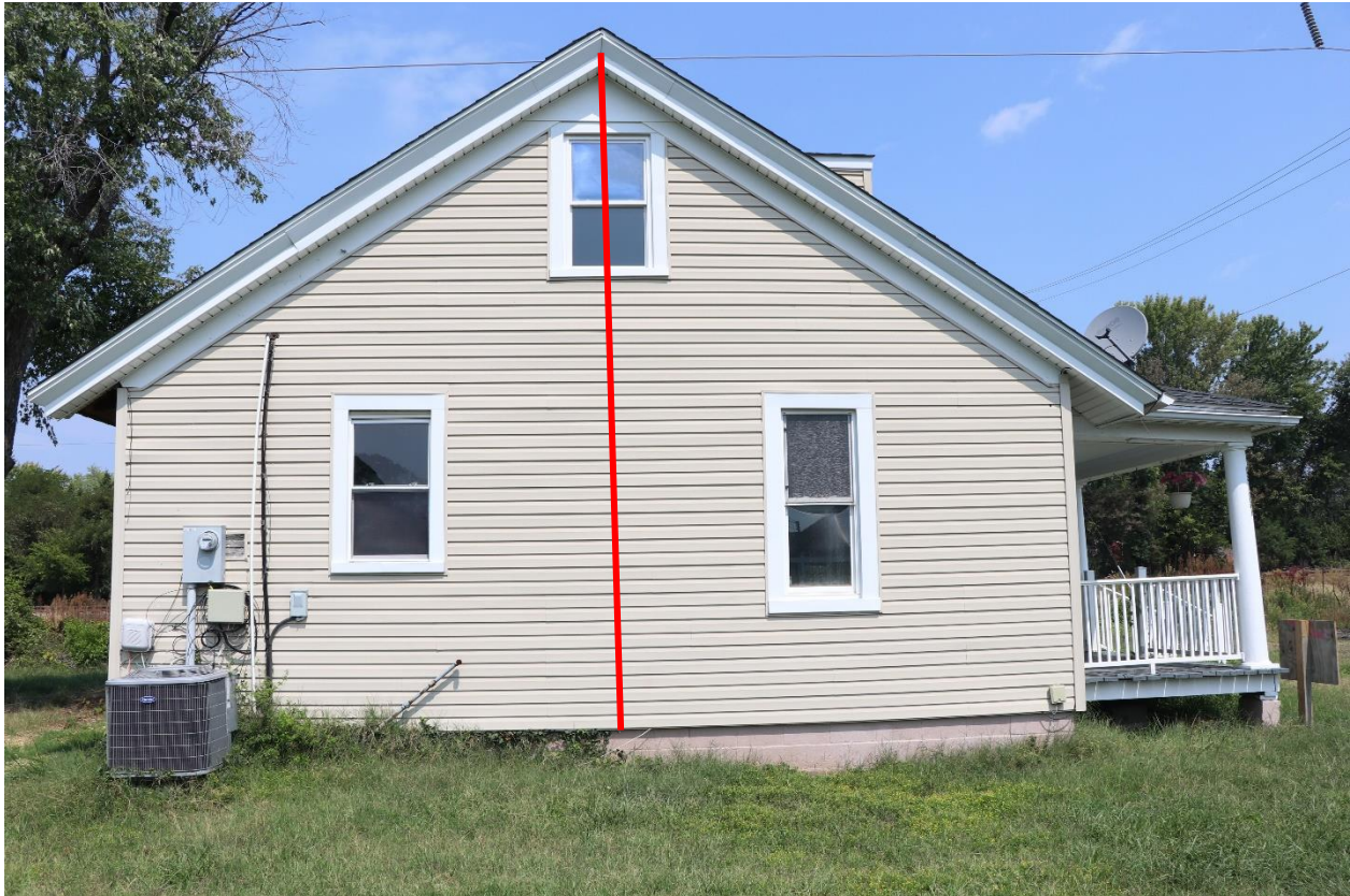
Figure 13. WJE measured the building height to the roof eave (red line) to 19-feet.
