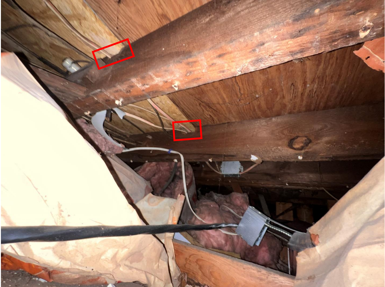
Figure 33. The Second Level floor joists were notched (red boxes) to accommodate electrical and other conduits.
