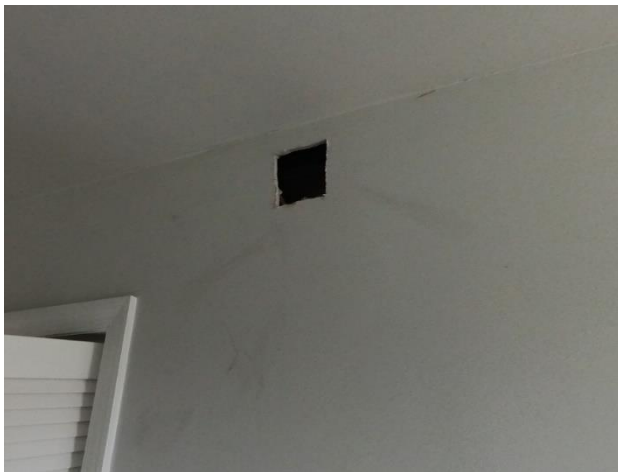
Figure 7. WJE conducted inspection opening 3 in the First Level hallway wall to observe the framing.
