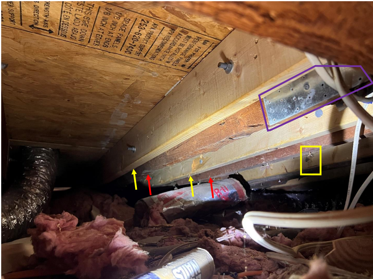
Figure 32. The original Second Level floor joists (red arrows) at inspection opening 4 were sistered with newer dimensional lumber bolted to the existing joists. The new lumber was marked with grade stamps (yellow box). Connections were strengthened with metal plate connectors (purple box).
