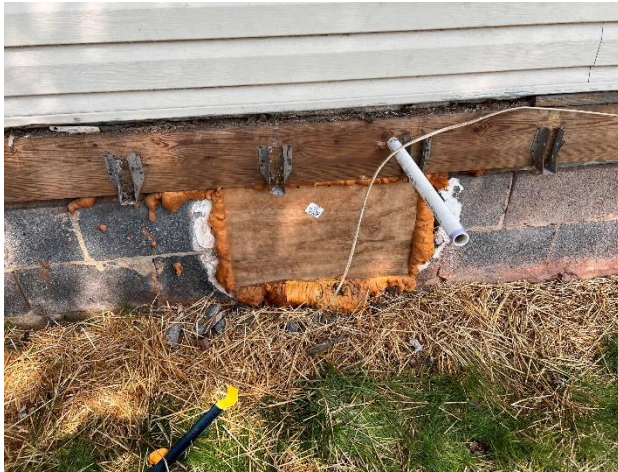
Figure 5. WJE removed the plywood and spray polyurethane foam covering the crawl space (inspection opening 1) to observe the First Level floor framing.
