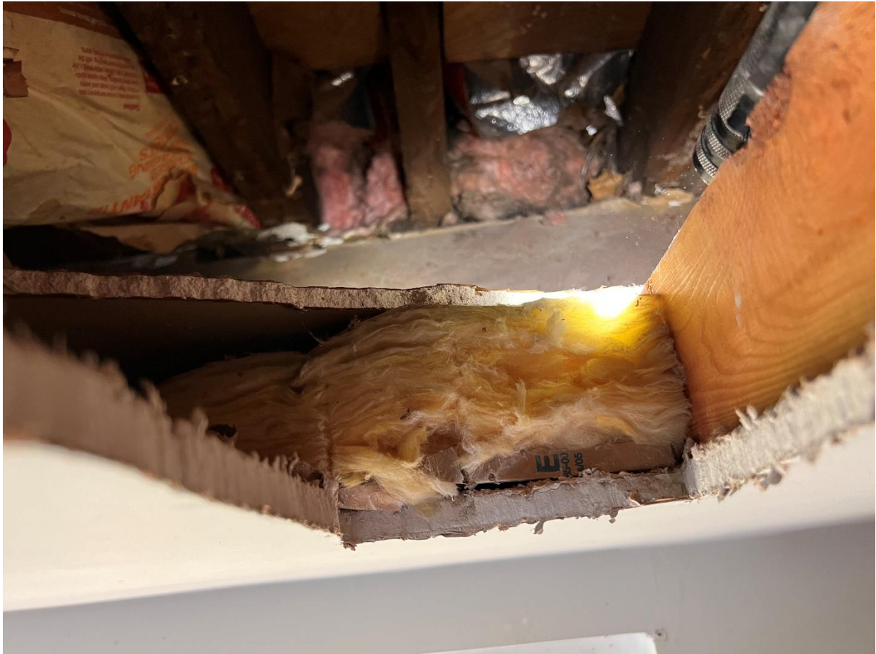
Figure 29. The First Level gypsum wallboard ceiling is suspended from the Second Level floor joists. Fiberglass insulation infills the joists on top of the gypsum wallboard ceiling.
