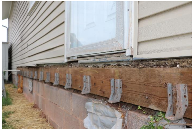
Figure 16. WJE observed the remaining joist hanger supports at the recently demolished back porch.
