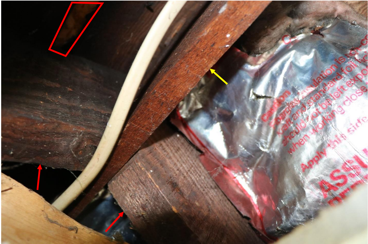
Figure 30. OSB was installed over wood planking (red box). The roof rafters (red arrows) frame into a central ridge beam (yellow arrow).
