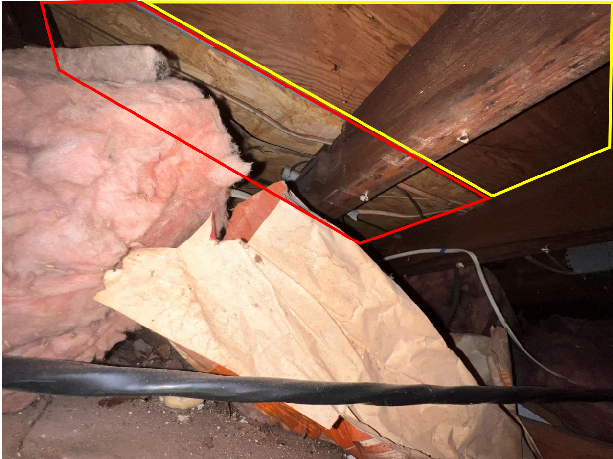
Figure 34. The Second Level sub-floor consisted of newer oriented strand board (red box) and older plywood (yellow box) sheathing.
