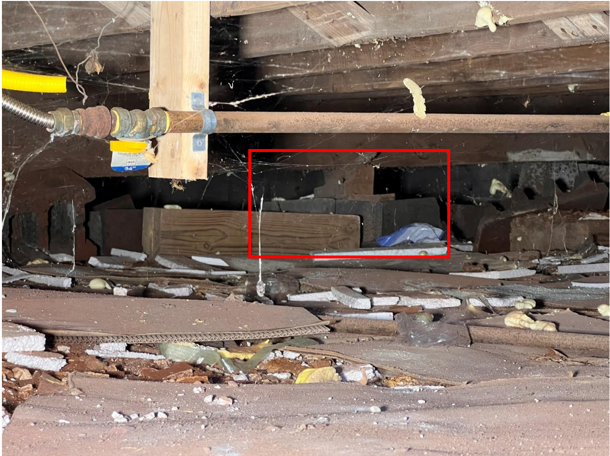
Figure 23. The central load bearing wall was supported by CMU blocks and wood posts (red box).
