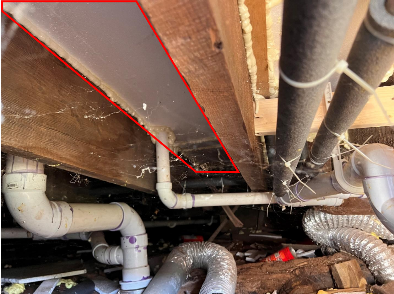
Figure 27. White rigid insulation (red box) was attached to the First Level sub-floor.
