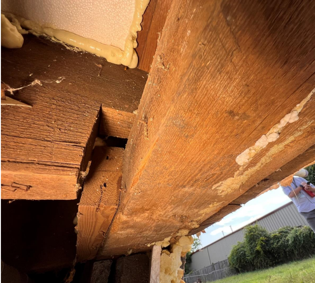
Figure 26. The First Level floor joist ends were notched and bear on a wood sill plate.
