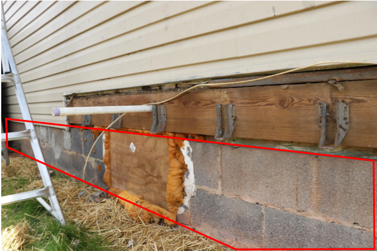
Figure 22. Exterior Cottage walls bear on a hollow CMU block foundation wall (red box).
