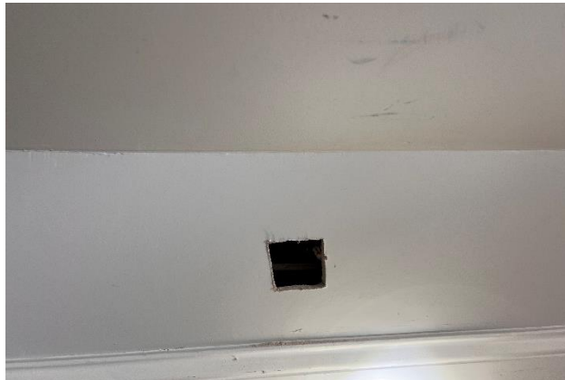
Figure 10. WJE conducted inspection opening 6 in the Second Level wall to observe the roof.
