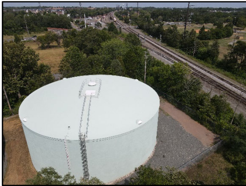
Dean Drive Storage Tank
