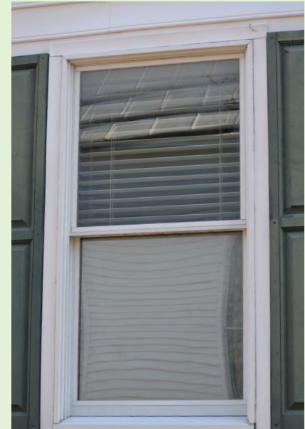
Vinyl windows are not appropriate for Contributing and Landmark structures.
