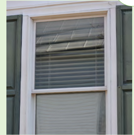
Vinyl windows are not appropriate for Contributing and Landmark structures.
