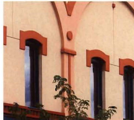
Required: Whenever stucco (EIFS) is used as an exterior material, details shall be introduced into the surface design to provide interest and surface variation.
