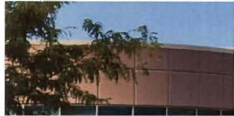
Required: Whenever stucco (EIFS) is used as an exterior material, surface texture must be incorporated in the form of scoring where no surface component exceeds 64 square feet in area.
