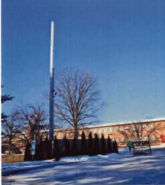
Figure 17.45.180: Monopole with internal antenna array
