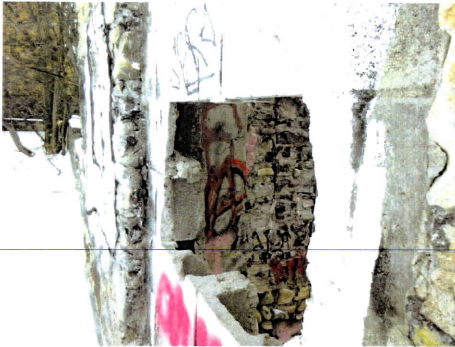
Photo 2 Damaged CMU masonry infill
