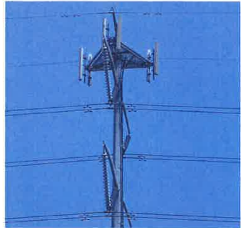
Stealth Design on Existing Utility Poles
