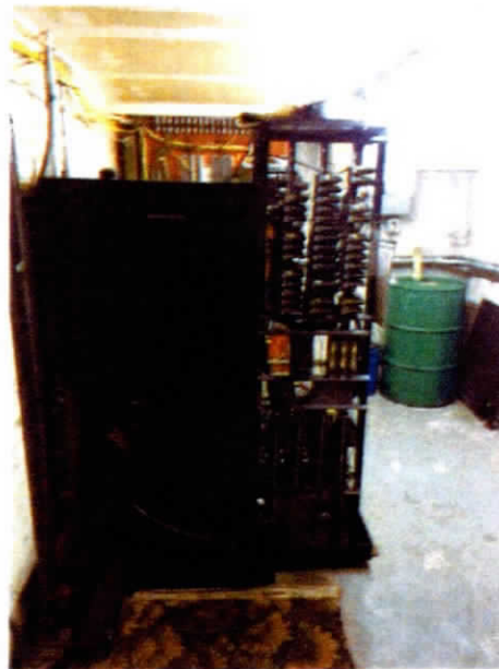
Figure S-27 Building 59 Elevator Pump and Oil Tank.
