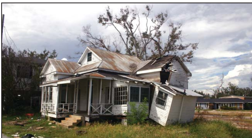
Hurricane Katrina damage in Bay St. Louis, Mississippi
