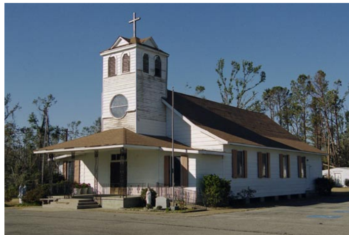
Figure 49. St. Stephen's Catholic Church received some cosmetic damage from Hurricane Katrina. Source: Michael Curtis.
