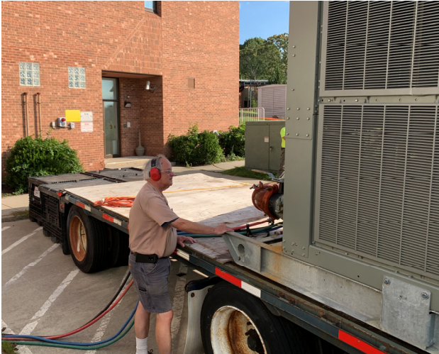
Skilled Building Technician Dave Smith inspects the portable chiller used during the Police Department AC failure. Dave has been with PWD for an impressive 43 years! Thanks Dave!
