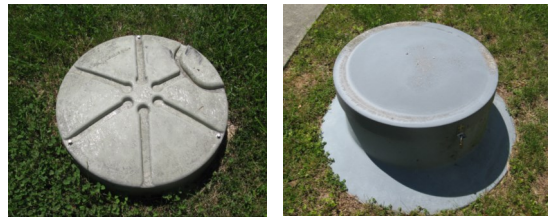
Exterior Grinder Pump Lids
