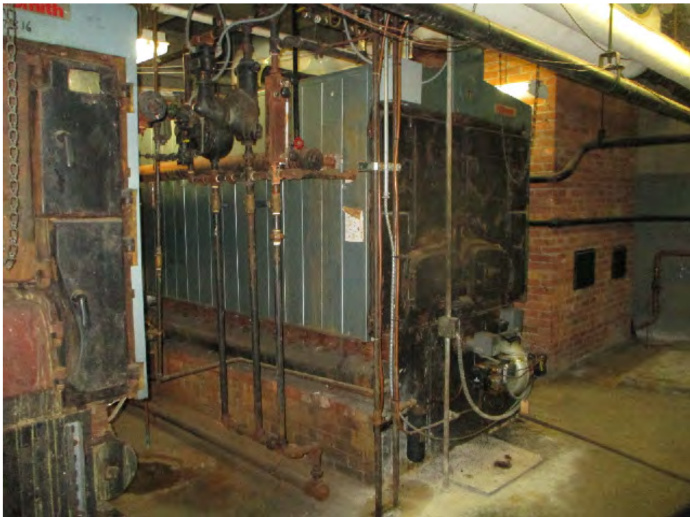
BUILDING NO. 1 - INTERIOR VIEW / MECHANICALS
