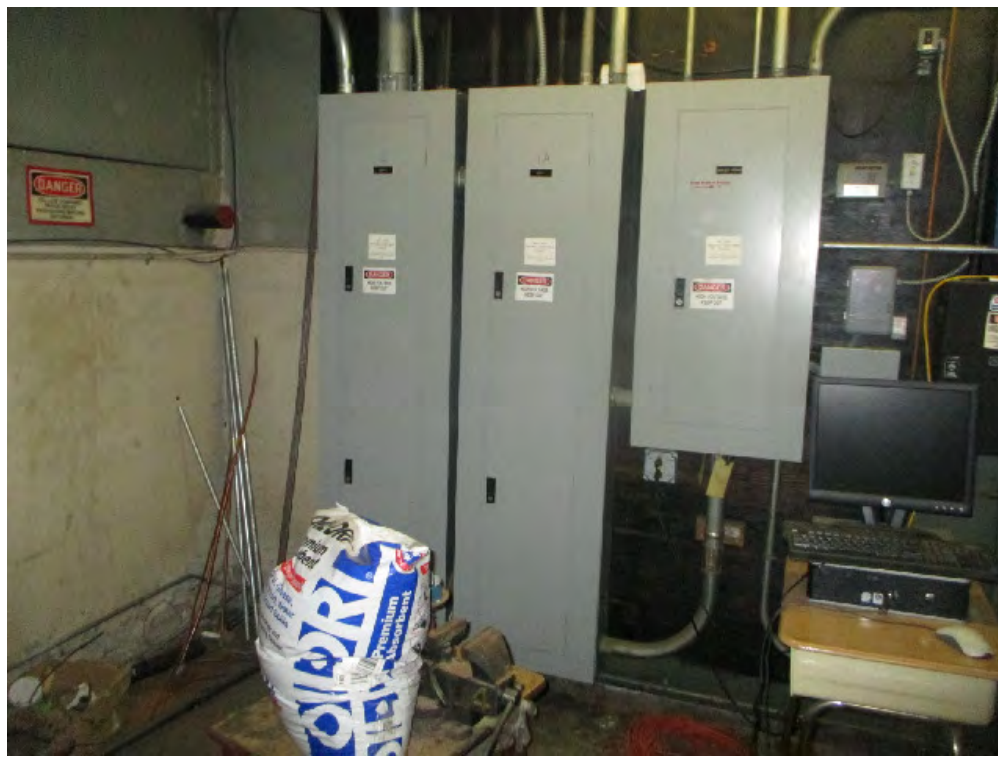
BUILDING NO. 1 - INTERIOR VIEW / MECHANICALS
