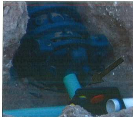
INCORRECT: BOTTOM PORT
