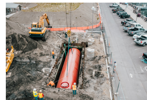
New fuel tanks were recently installed.
