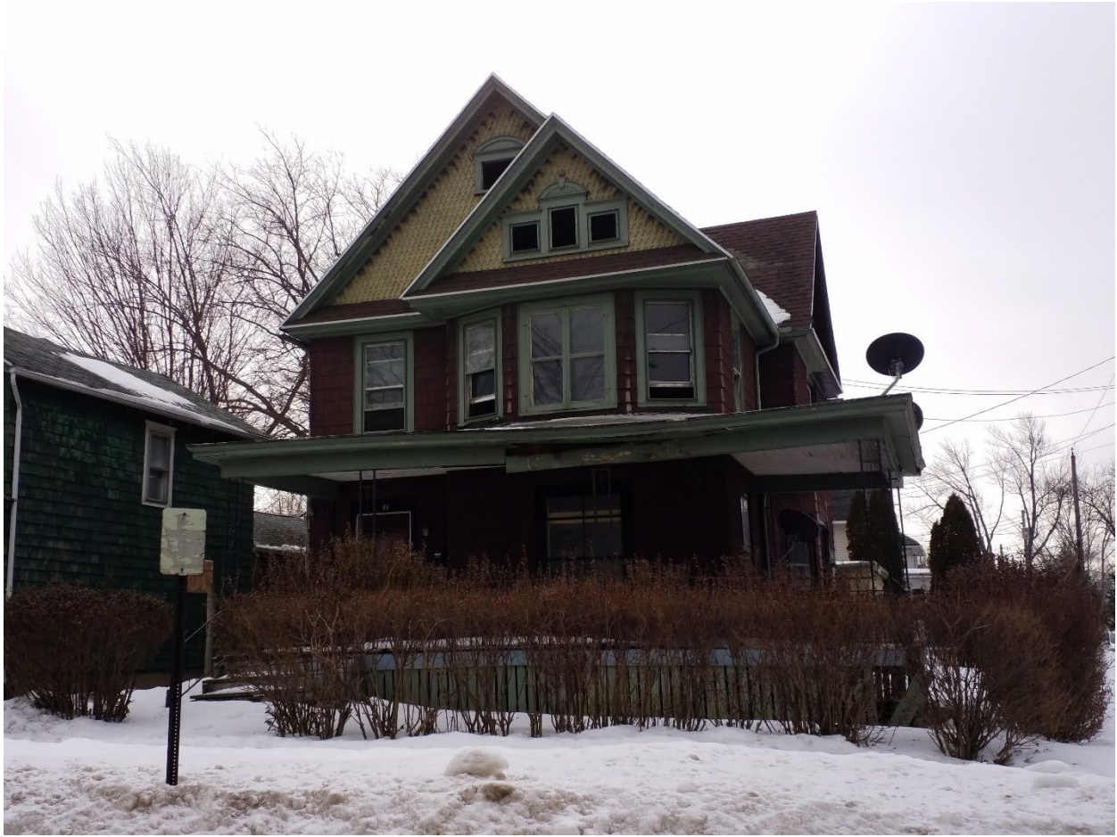
65 East Sixth Street: 2 story frame two family on basement with attached garage. Partially Fire Damaged
