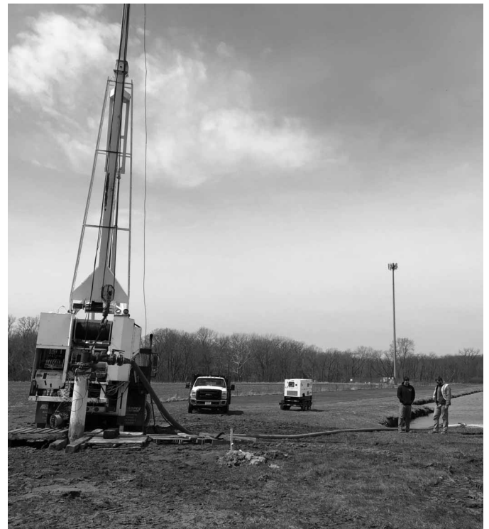
Des Moines Water Works worked with the U.S. Geological Survey in 2022 to evaluate how to collect raw water along the Des Moines River. This included test wells that were drilled and pumped, shown here, at our Saylorville Water Treatment Plant. The data gathered will help to aid in the design of the Saylorville Plant expansion. The cost of initial design work is included in the 2023 budget.
