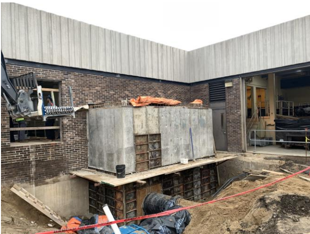
Photo 5: Grit Building Influent Chamber
