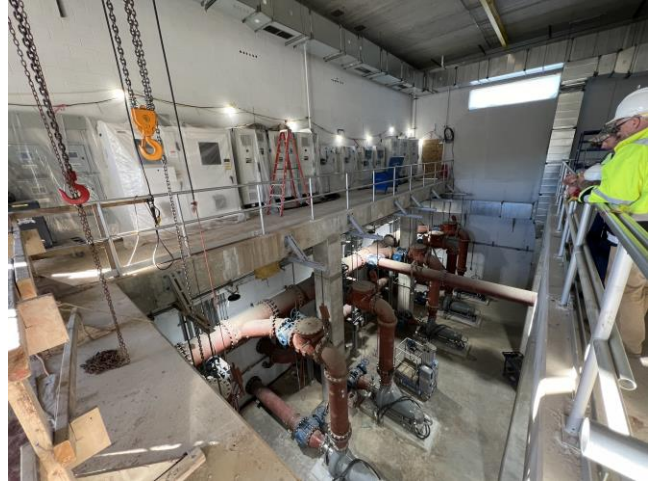
Photo 8: Headworks Building Pump Room
