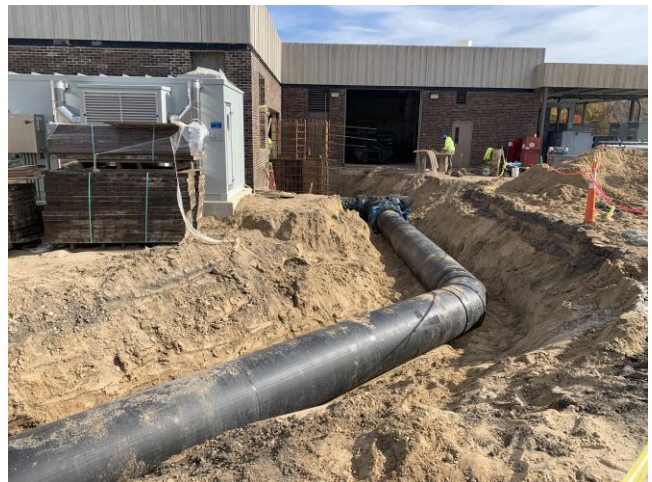
Photo 6: Grit Building Force Main Bypass
