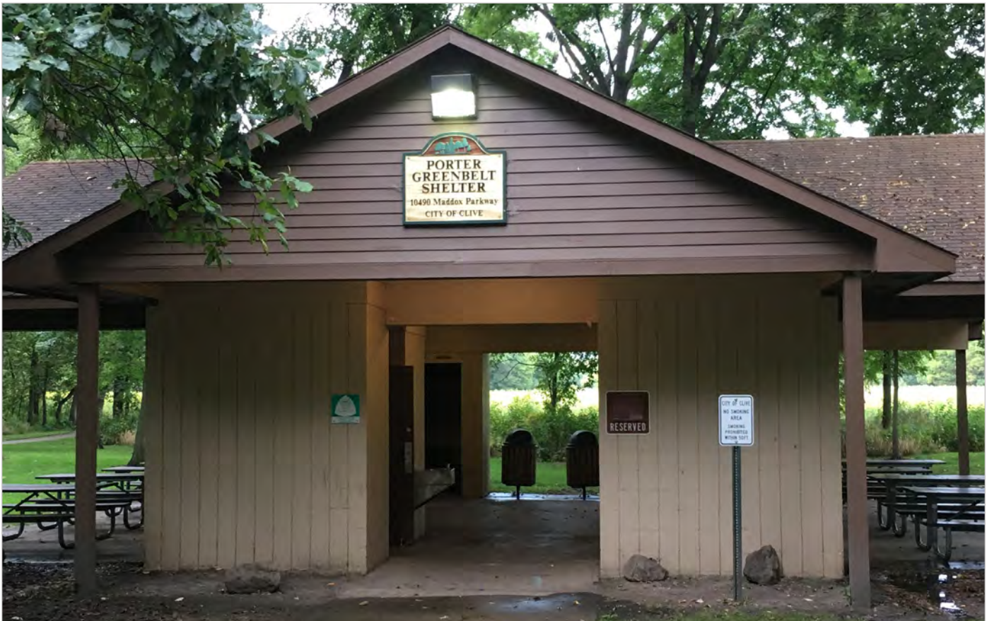
In 2015, significant rainfall within Walnut Creek Watershed caused flooding within the Greenbelt. Porter Shelter is located within the floodway and should be relocated as it is nearing the end of its design life.
