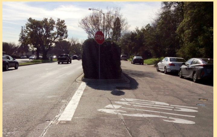
Missing sidewalk at Huntington Drive frontage road
