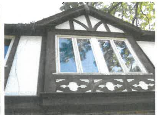
Large dormers with rough stucco and half timbering details, and replaced window frames, north elevation
