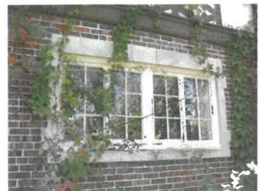
Six lite, steel casement windows
