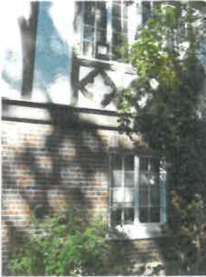
Detail of typical materials at coach house: red variegated brick, rough plaster stucco with decorative half timbering, and multi-paned steel casement windows
