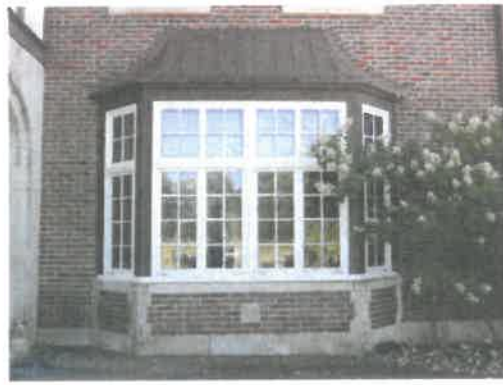
Hooded bay window at the north elevation, just west of the porte cochere
