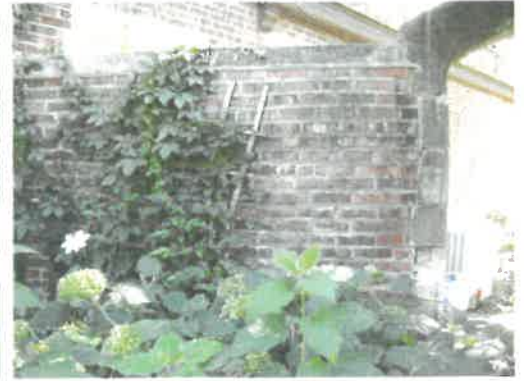
Joint failure at the garden wall
