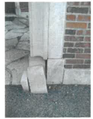
Base of the stone arch opening at the porte cochere, showing damage
