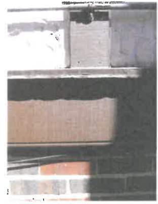
Detail showing typical materials at coach house: red variegated brick, rough textured stucco with decorative half timbering
