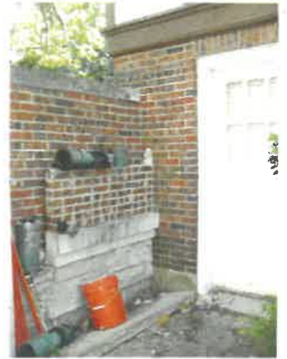
Detail of wood panel door leading into garage space at coach house
