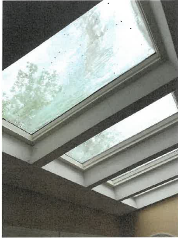
Skylight seals broken
