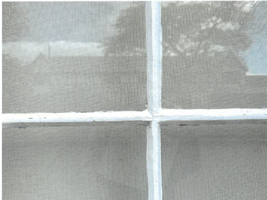
Photo 9 - Example of deteriorated glazing putty in October of 2024.
