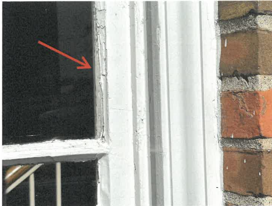
Photo 8 - Example of deteriorated glazing putty in October of 2024.
