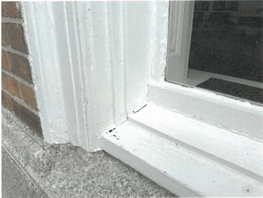
Photo 6 - Example of deterioration at Window Type F in October of 2024.
