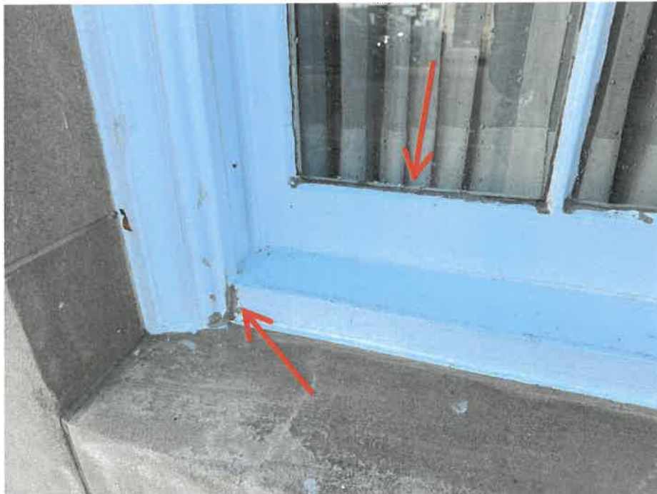
Photo 7 - Example of deterioration at Window Type B in October of 2024. Arrow points to sealant applied after painting was done.
