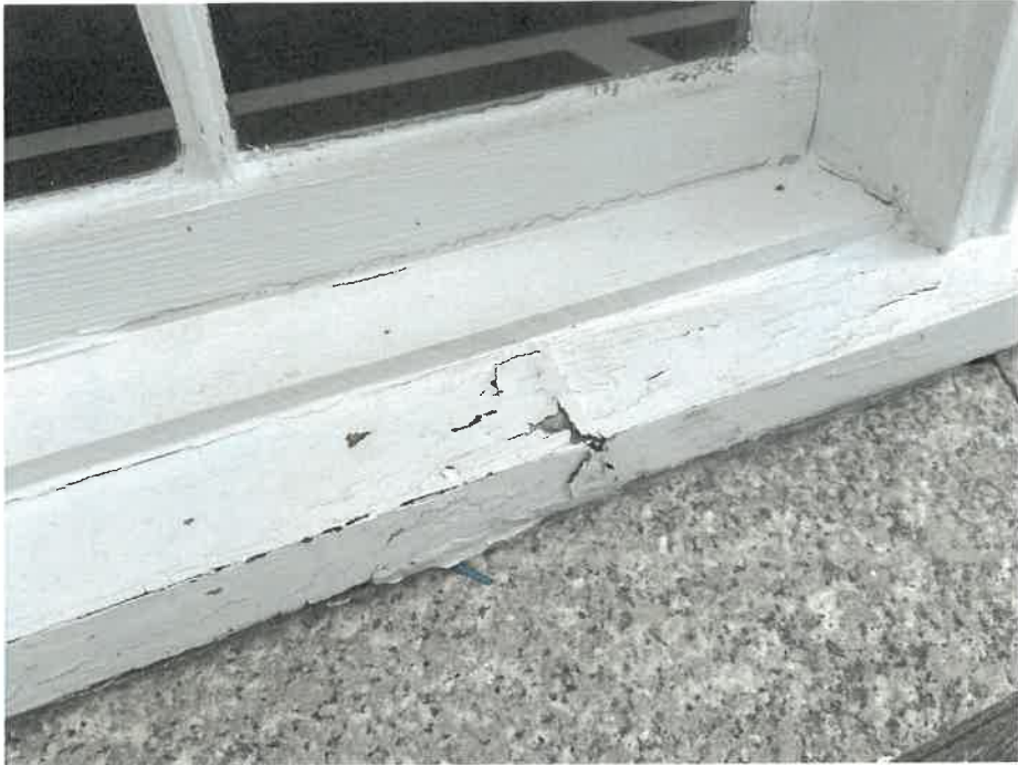
Photo 4 - Example of deterioration at Window Type F in October of 2024.
