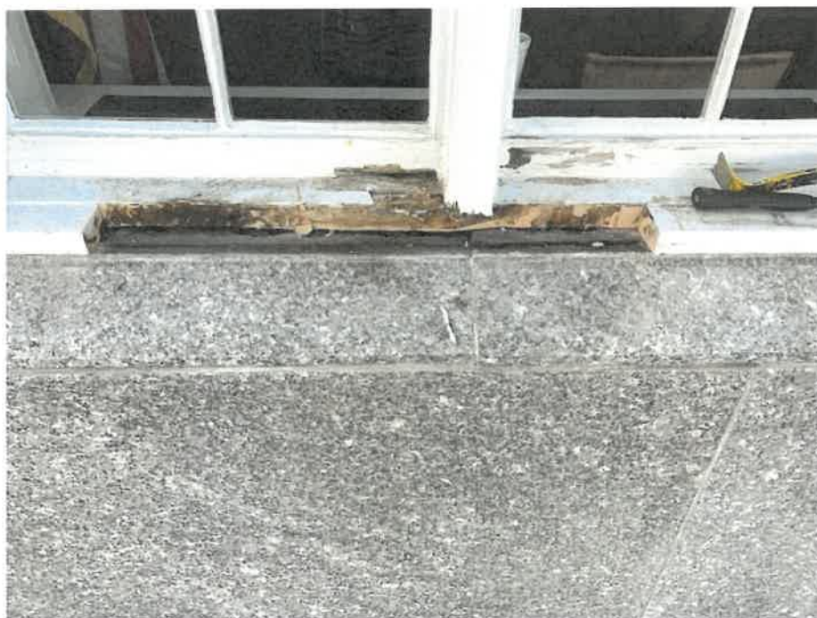
Photo 3 - View of deterioration at Window Type F in 2023 during repairs.
