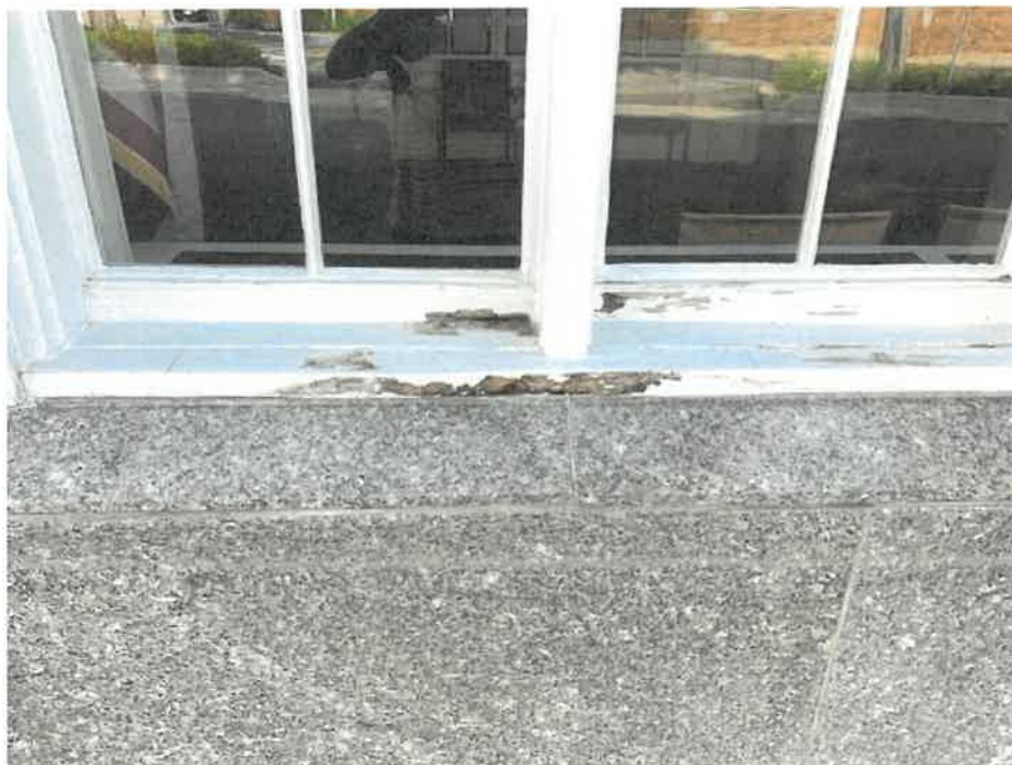
Photo 2 - View of deterioration at Window Type F in 2023 prior to repairs.
