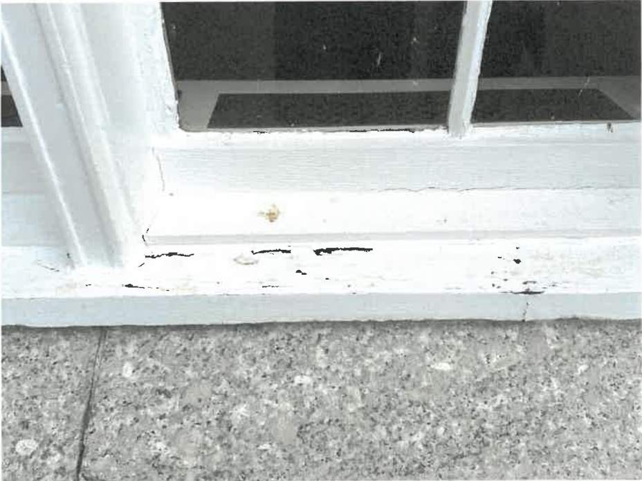
Photo 5 - Example of deterioration at Window Type F in October of 2024.
