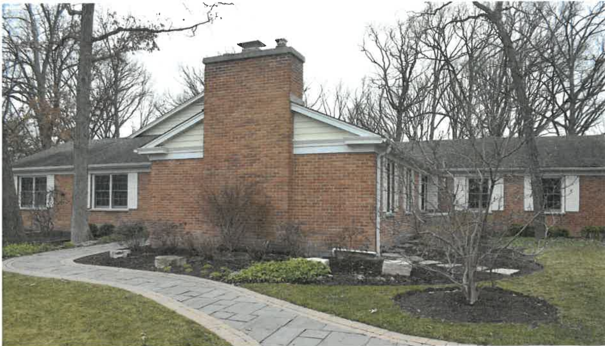
Photo No. 1 – Front of residence. Note proximity of trees to residence. The roots of trees close to a residence can cause foundation wall damage.
