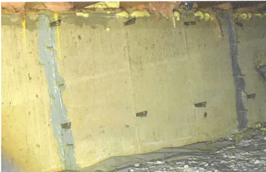
Photo No. 4 – Typical foundation crack repaired in the crawl space. No “re-cracking” observed.
