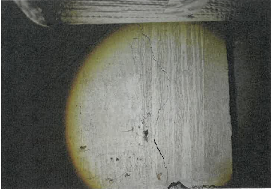
Photo No. 3 – Crack to be repaired at entry into crawl space at rear of property.
