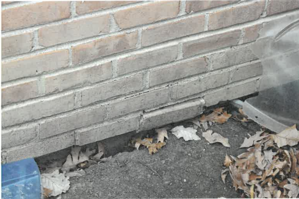
Photo No. 5 – On exterior of residence along the north basement foundation wall, note shifting of foundation wall inward. Brick, which is to bear on the foundation wall, is almost off its support. To a lesser extent, loss of foundation wall bearing was observed along the south and east sides as well.
