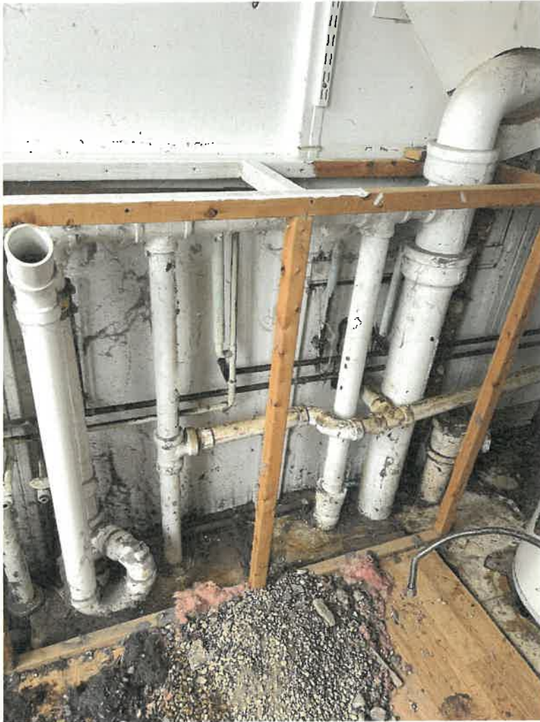
Existing Utility Room – Slab Construction – Significant Water Damage
