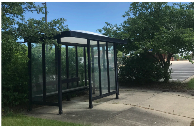
Photo of existing bus shelter on the west side of the train tracks.
