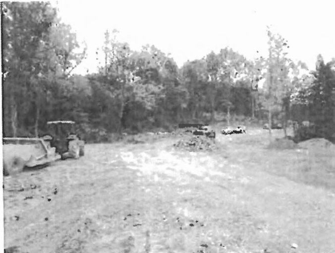
Photo 49 Staged equipment Orientation E
