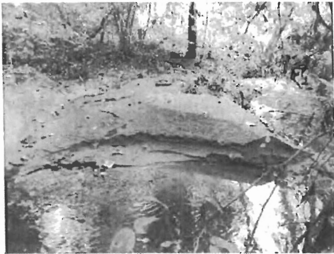
Photo 53 Dunker Creek with sediment observed Orientation SE
