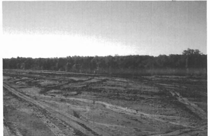
Fig. 8 Description: Evidence of land disturbance occurred. No ESC measures installed or observed.
