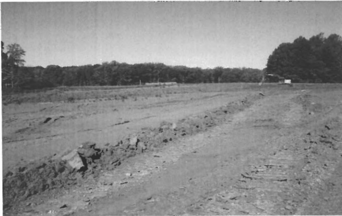
Fig. 7 Description: Evidence of land disturbance occurred. No ESC measures installed or observed.
