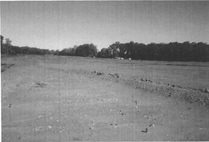
Fig. 5 Description: Evidence of land disturbance occurred. No ESC measures installed or observed.
