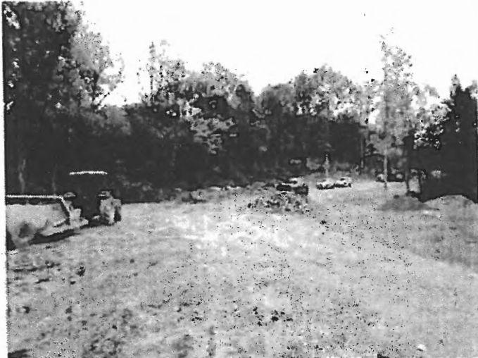
Photo 49 Staged equipment Orientation E
