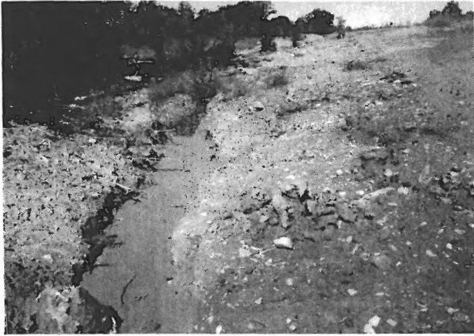
Fig. 9 Description: Evidence of land disturbance occurred. No ESC measures installed or observed.
