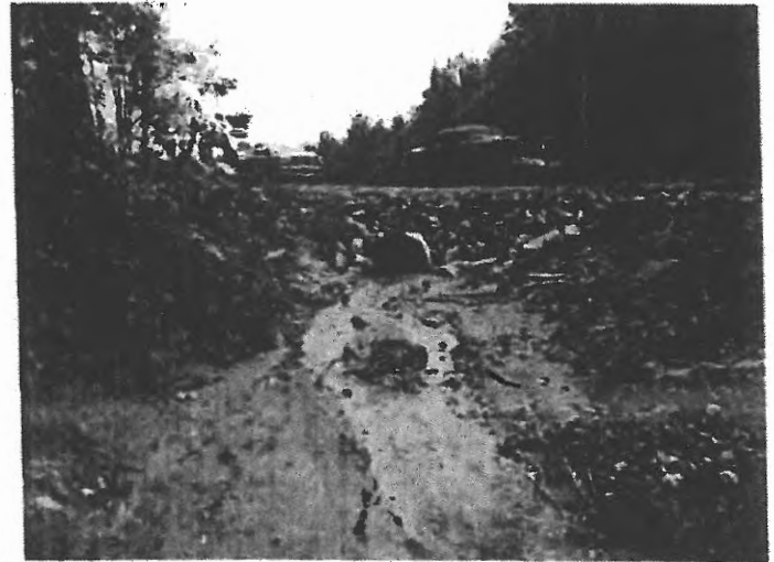
Photo 56 Recently construction stream crossing. Pipe is countersunk to an appropriate depth. Bank stabilization needed Orientation S
