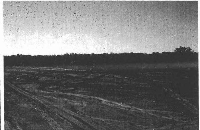
Fig. 8 Description Evidence of land disturbance occurred. No ESC measures installed or observed.
