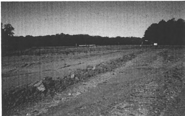
Fig. 7 Description: Evidence of land disturbance occurred. No ESC measures installed or observed.
