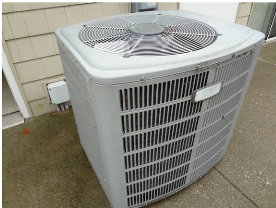
Photo #21: Condensing unit for community room
