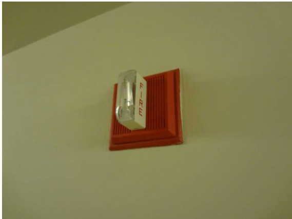
Photo #27: Strobes throughout buildings
