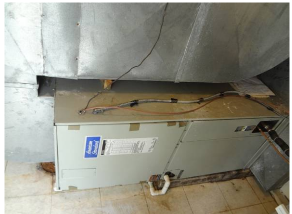
Photo #22: Air handler provides air conditioning for community room
