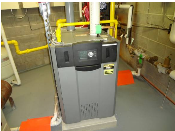
Photo #23: Domestic hot water boiler
