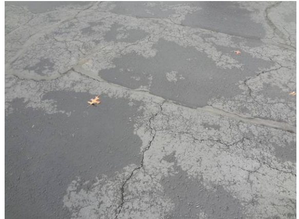
Photo #8: Asphalt paving shows signs of cracking throughout site
