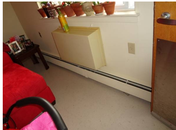
Photo #34: Baseboard heaters provide heat throughout building
