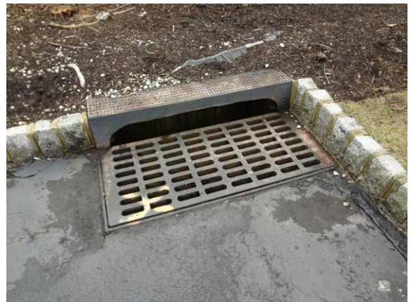
Photo #10: Catch basins throughout site collect water runoff
