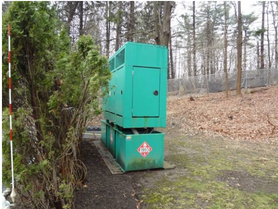
Photo #25: Backup generator
