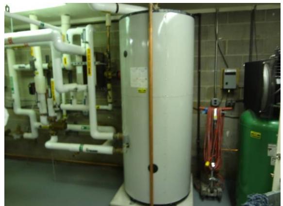
Photo #24: Indirect-fired water heater connected to domestic hot water boiler
