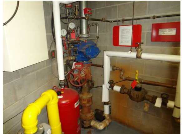
Photo #26: Dry-pipe sprinkler system
