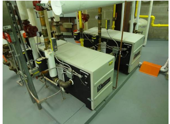
Photo #20: Heating boilers
