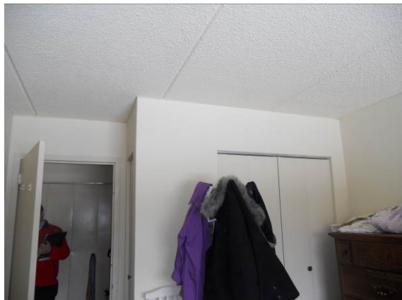
Photo #47: Apartment unit bedroom with no smoke detector
