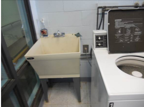
Photo #37: Laundry sink with non-GFCI
