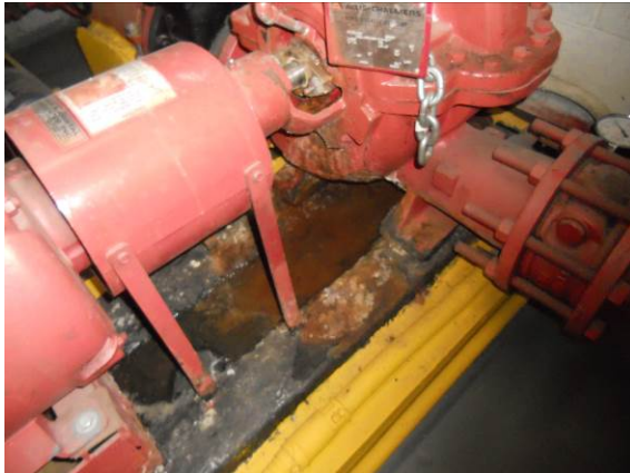
Photo #25: Fire pump with excessive corrosion at pan
