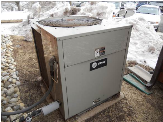
Photo #17: Condensing unit
