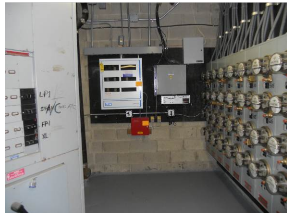
Photo #30: Fire alarm panel and electrical meter bank
