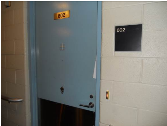
Photo #51: Apartment unit ADA entrance
