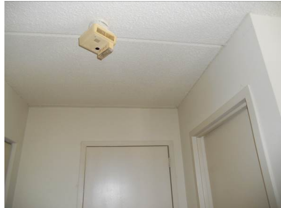
Photo #50: Apartment unit smoke detector and strobe just outside of bedroom
