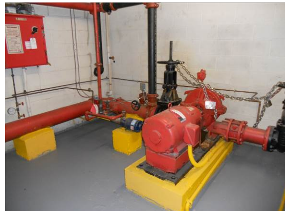
Photo #24: Fire pump
