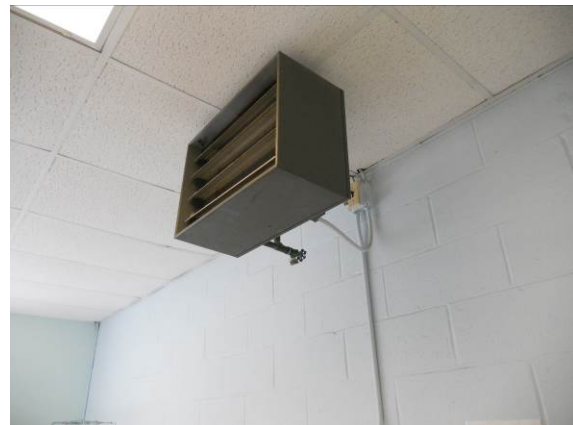
Photo #36: Unit heater in laundry room
