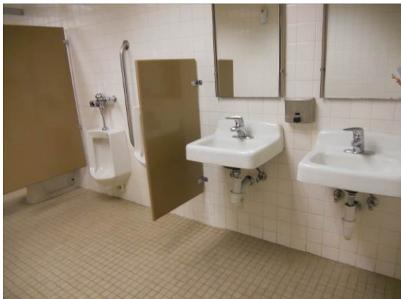
Photo #41: Common area men's restroom with loose drain pipe insulation
