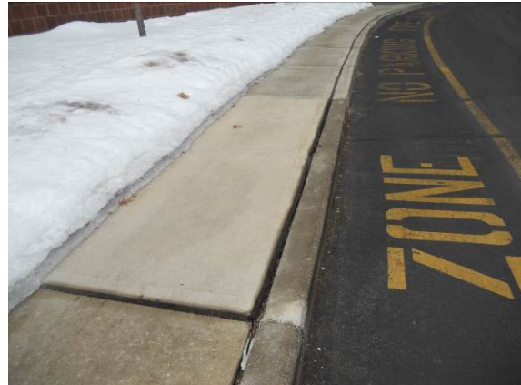
Photo #8: Shifted concrete walkway
