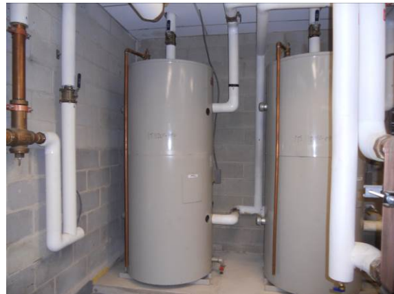
Photo #28: Domestic water storage tanks
