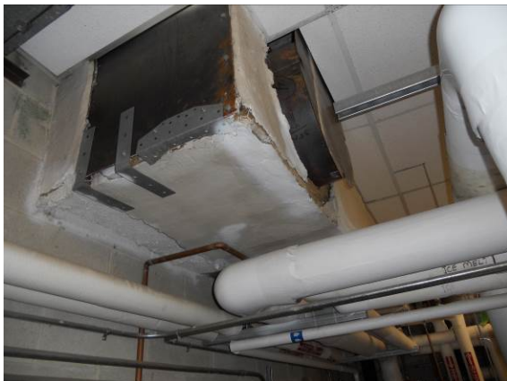
Photo #29: Suspect asbestos at duct
