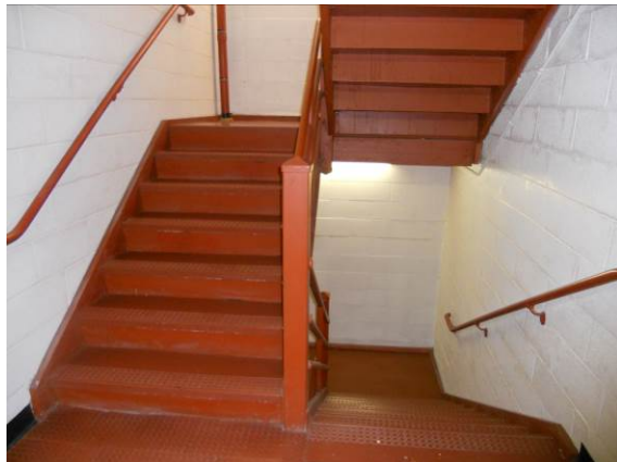
Photo #33: Fire stair without continuous inner railing but extensions on outer railing
