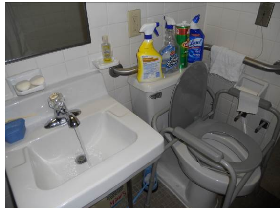
Photo #54: Apartment ADA unit with non-compliant faucet handle and grab bar lengths
