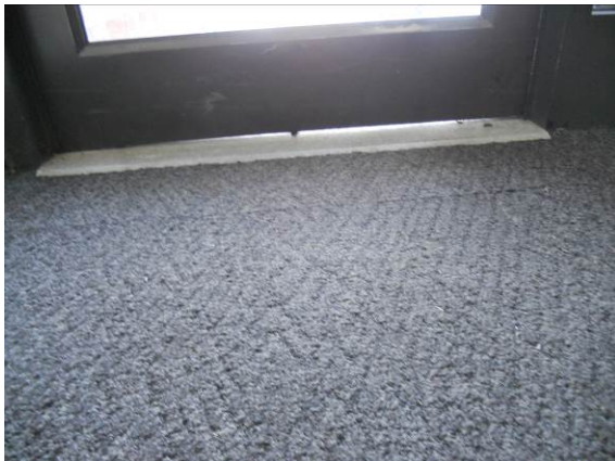
Photo #57: Secondary entrance with daylight seen under door frame
