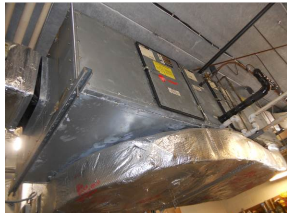
Photo #18: Air handling unit
