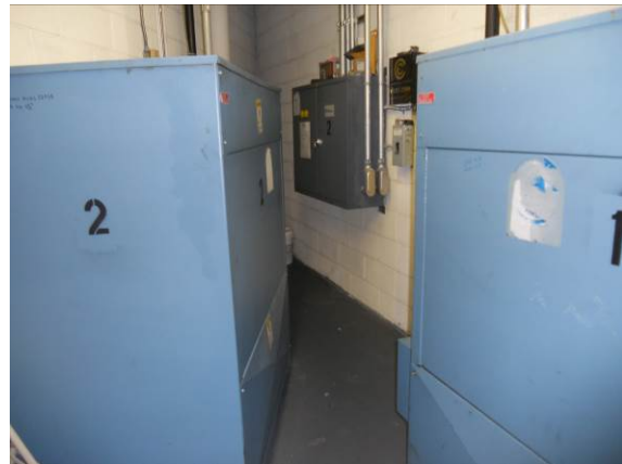
Photo #22: Elevator machinery
