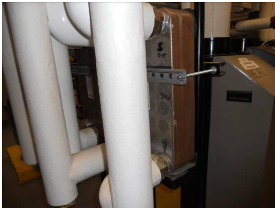
Photo #27: Flat plate heat exchanger
