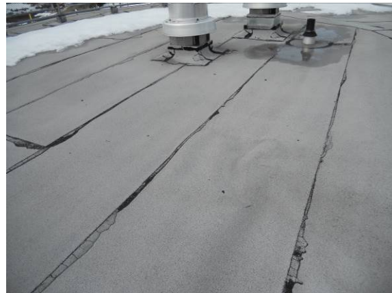
Photo #16: Roof close up showing bulges in membrane
