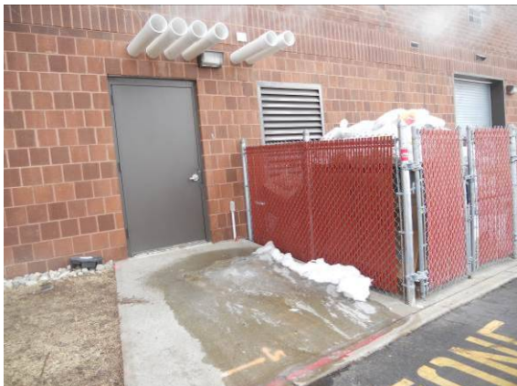
Photo #11: Condensation exhaust causing ice to form at exit from main mechanical room
