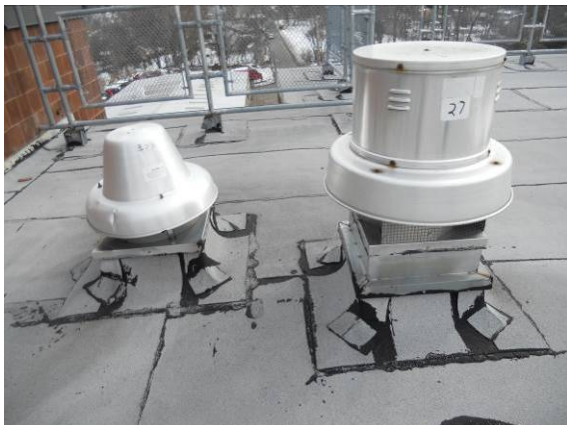
Photo #23: Exhaust fans
