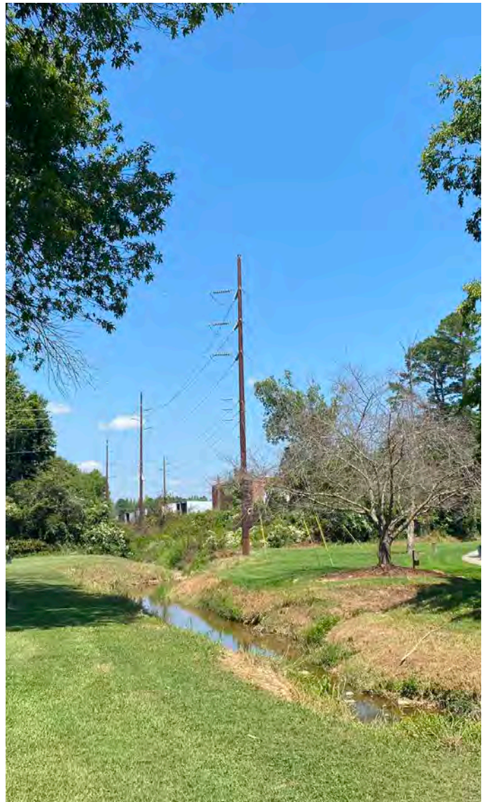
Transmission lines along Hasketts Creek
